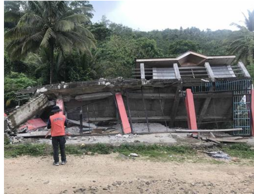
Totally collapsed house in Brgy. Sto. Nino, Makilala
