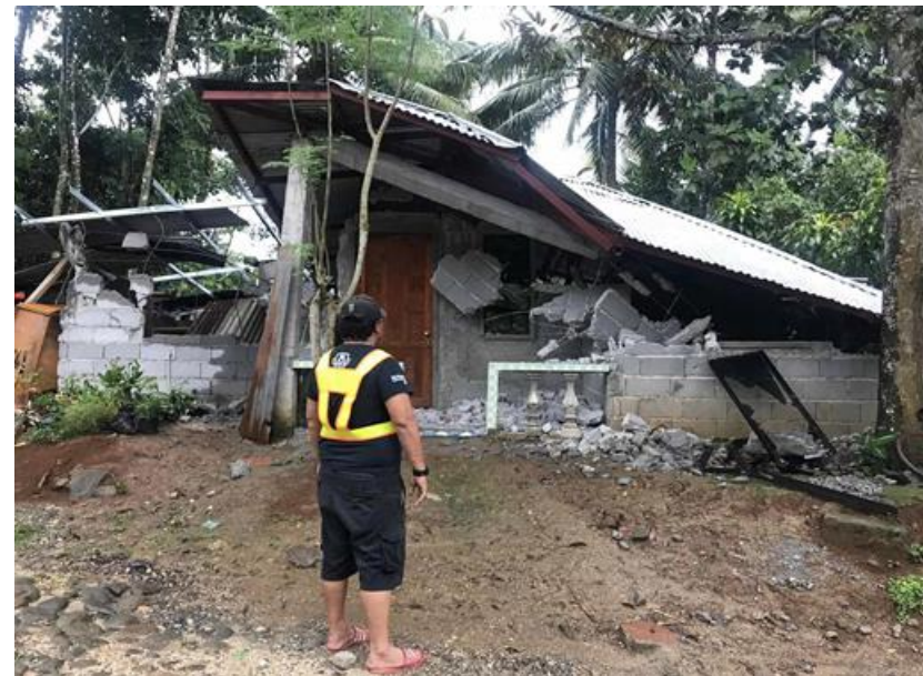
Totally collapsed house in Brgy. Kisante, Makilala
