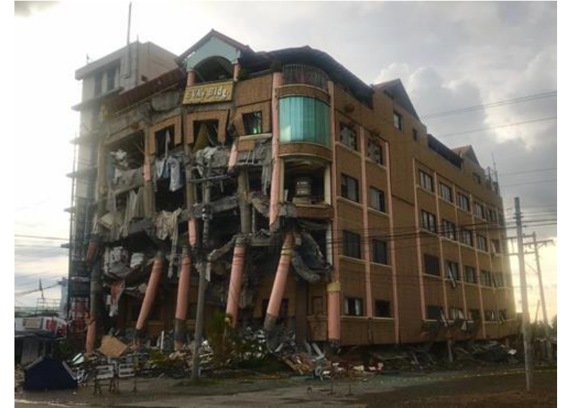
Eva's Building damaged during the October 31 2019 M6.5 event. Photo by the PHIVOLCS QRT (10312019)
