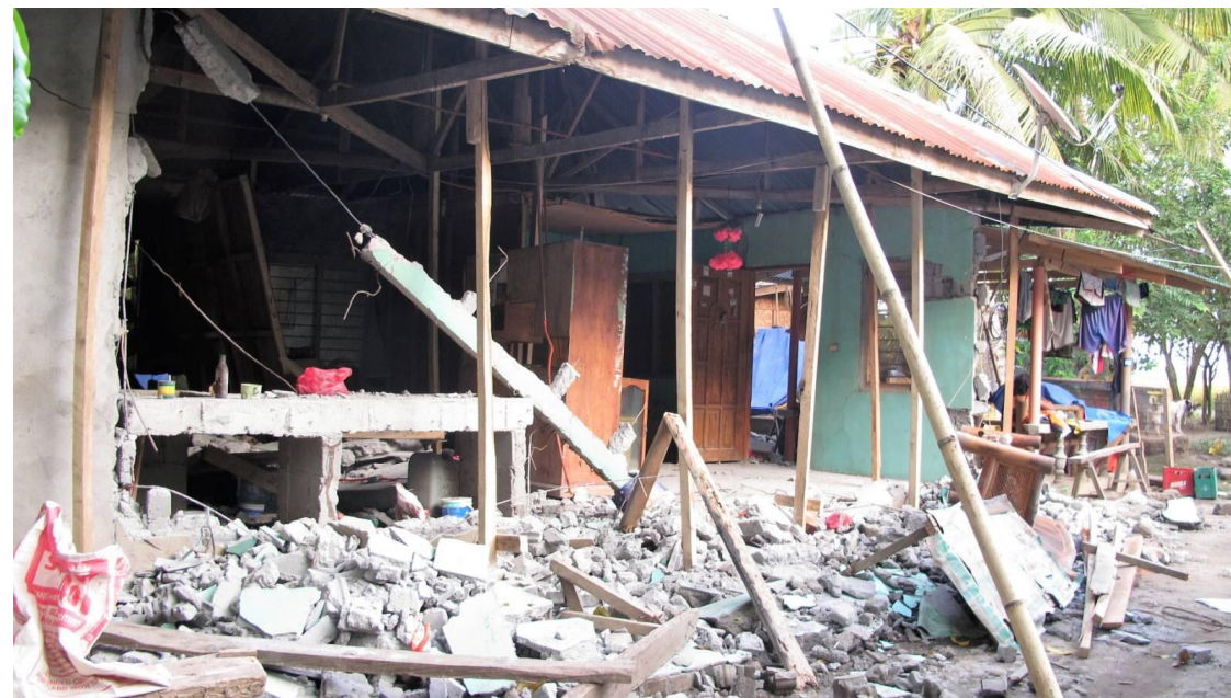
Totally collapsed wall of a house in Brgy. Bagontapay, M'lang (lumber post were installed post-shaking to prevent total collapse of the roof)
