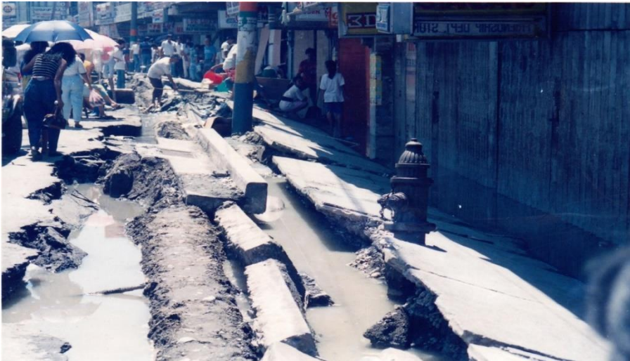
Underground utilities rising to the surface in Dagupan due to the 1990 Luzon earthquake
